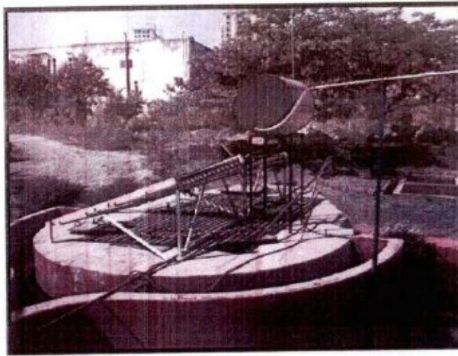
A Typical Pre-Digester
